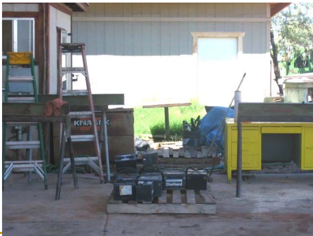
Batteries palletized, sheltered
